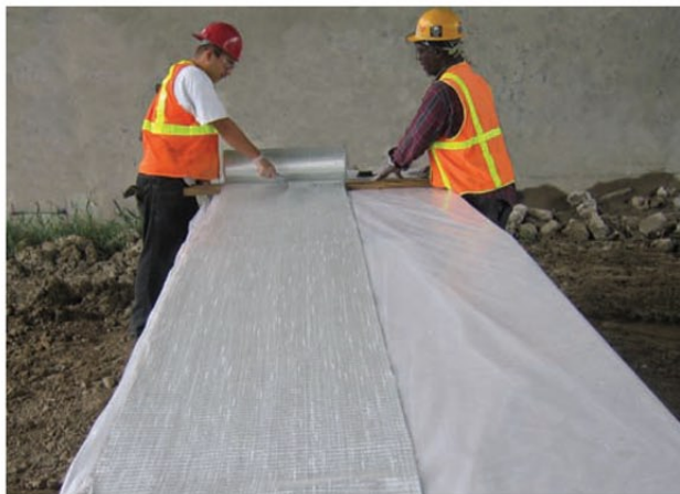
Figure 4: Cutting of GFRP fabrics is simple and can be achieved on site.
