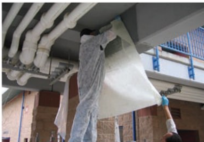
Figure 2: Shear strengthening of ends of beams in a pedestrian bridge with glass-fibre-reinforced polymer (GFRP) fabric.
