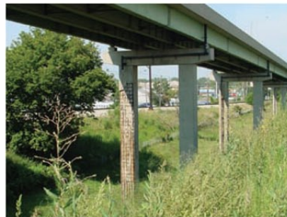
Figure 3: Corrosion of reinforcing bars in a bridge pier.
