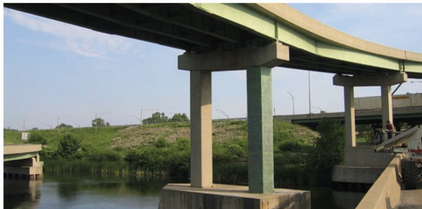
Figure 6: The finished bridge, showing the wrapped column on the right and the unwrapped column on the left.
